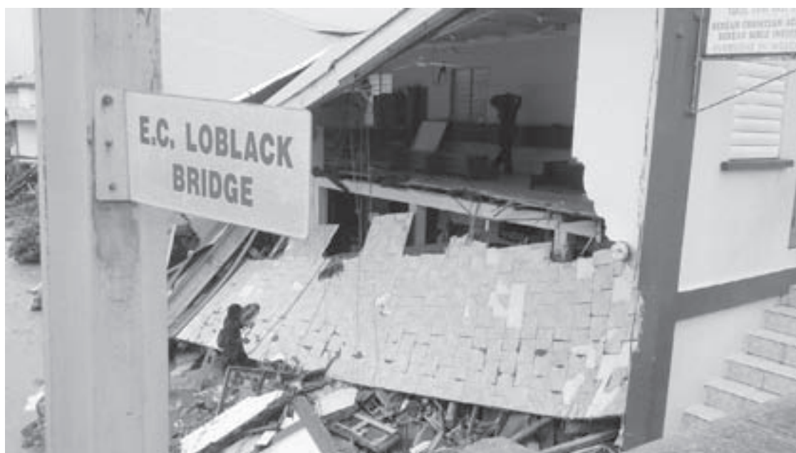
The Beran protestant church is partially collapsed due to Tropical Storm Erika in Roseau, Dominica. Rescue teams worked Sunday to reopen roads to remote communities in Dominica after Tropical Storm Erika caused flooding and mudslides that killed at least 20 people and left more than 50 missing on the Caribbean island.
